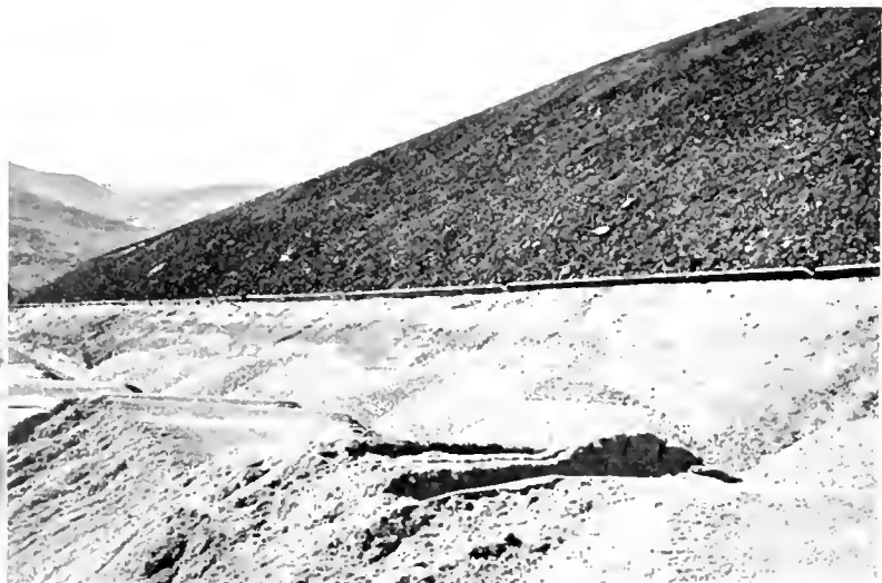
Finished 1:1 slope too smooth to retain lumpy adobe top soil. Header-board above plant mix ditch line to hold cover soil
